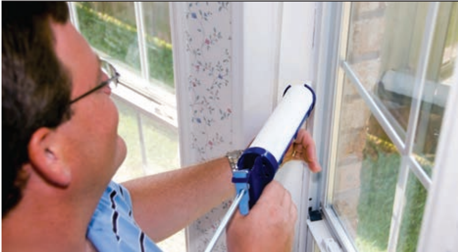
If you feel a temperature change around a window or door, seal the perimeter with caulk.
